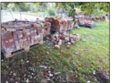
Photo of salvaged bricks from collapsed wall cleaned and ready to be used to rebuild the wall.
